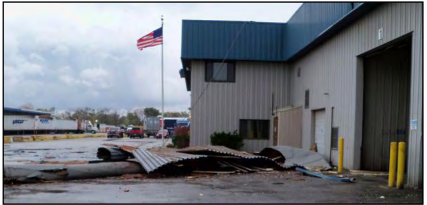
Record-setting windstorm damaged the roof at the Markham, IL terminal.
